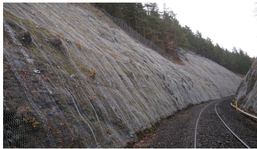
Metal netting to secure rock slope. (Source: https://www.externalworksindex.co.uk )
